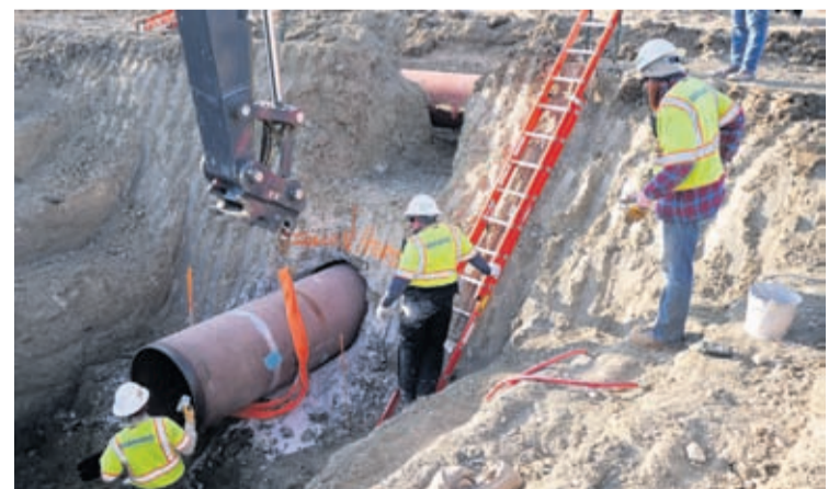
In this April 13, 2020, photo provided by TC Energy, construction contractors for TC Energy are seen installing a section of the Keystone XL crude oil pipeline at the U.S.-Canada border north of Glasgow, Mont.
